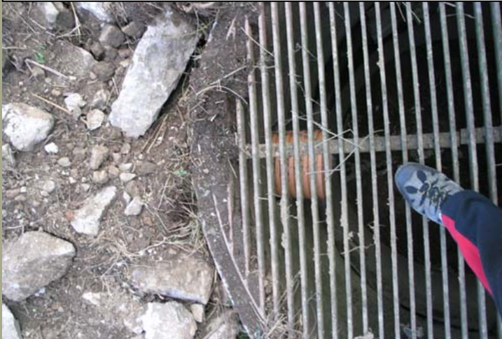
OUTLET FROM WASTE-WATER TREATMENT PLANT
